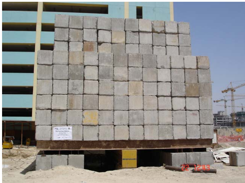
Figure 3.1: Kentledge (concrete blocks as dead load) of the single pile, D = 75 cm
